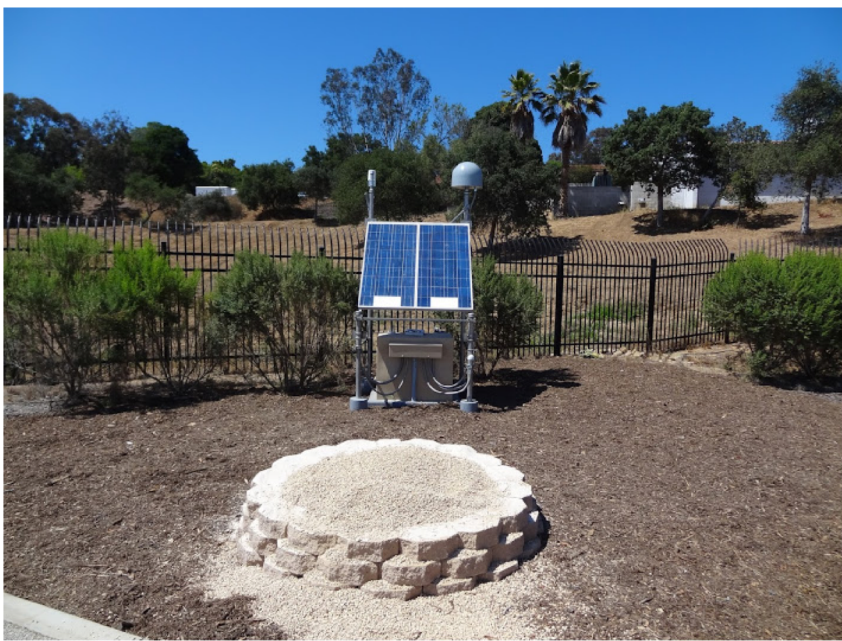
Figure 2. Station EOCG at the Santa Barbara Emergency Operations Center. Seismic vault is located in the foreground. Photo courtesy of Dan Determan, USGS. Photo was taken sometime between July and December 2014.
